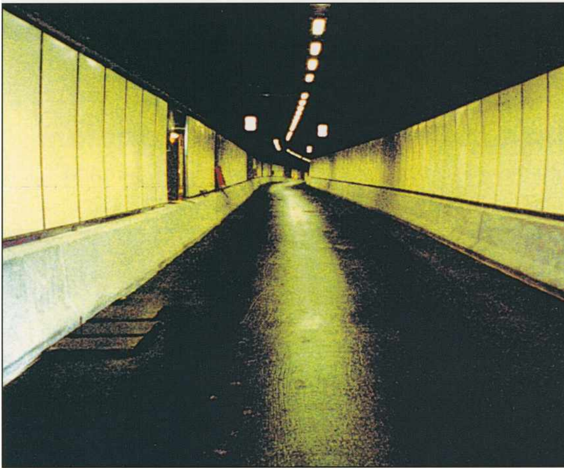
Sydney's long awaited Eastern Distributor road network included a series of tunnels connecting the Eastern part of the city with the Airport and beyond. Over 100,000m 2 of pavement had to be treated in quick time. The SAMI team worked both day and night shifts to meet deadline.
