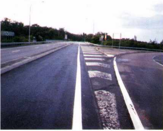
The HIPAR dense grade pavement (left) and the original deteriorated open grade pavement (right).
