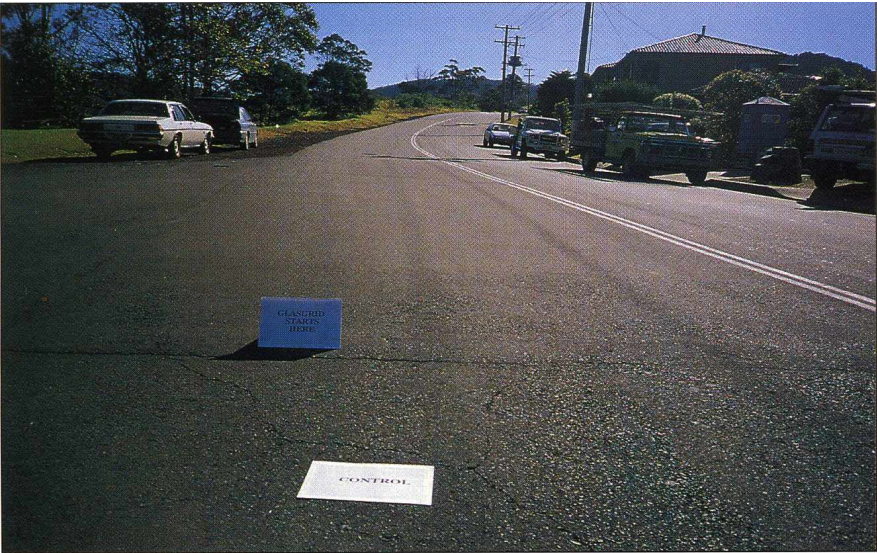
O'Briens Road, Figtree: Note the cracked control section in the foreground, with the GlasGrid reinforced area immediately behind.
